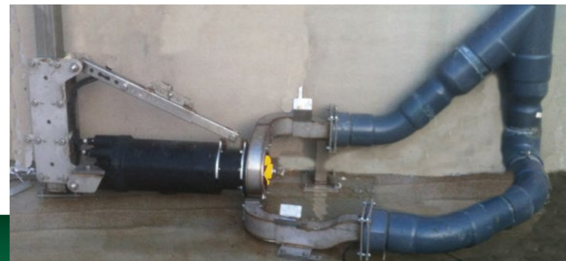
B3TR Jet with pumping device
